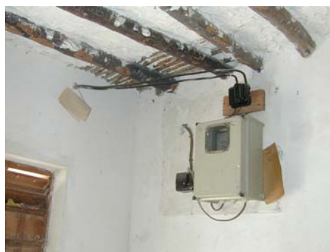
Electric meter inside a private home (Uroa 2001)
