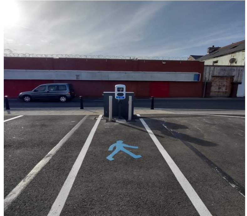
A DCC EV charge point
